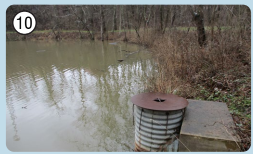
EXISTING CONDITION TEN
