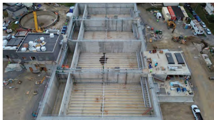
WPCP construction photo from mid-2024, showing the Headworks Building, S.B.R. tanks, and Disinfection Building (from left to right).
